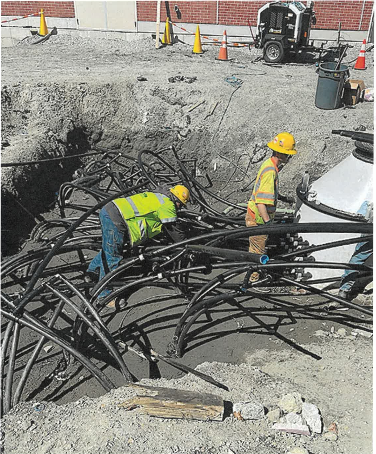
A crew ties loops together at a manifold vault beneath the Farley lot pump house location in Framingham, Massachusetts. Images courtesy of Eversource Energy.
