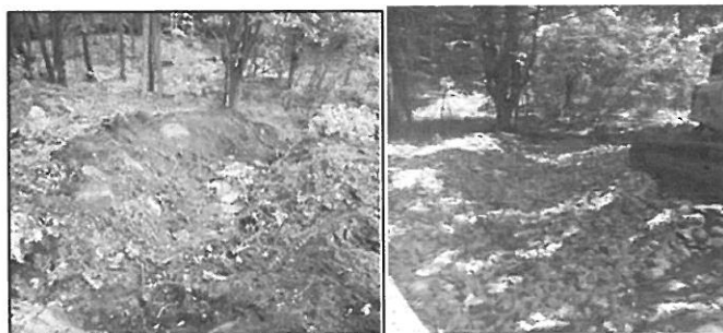
Actively eroding outfall (L) and newly stabilized channel (R).
