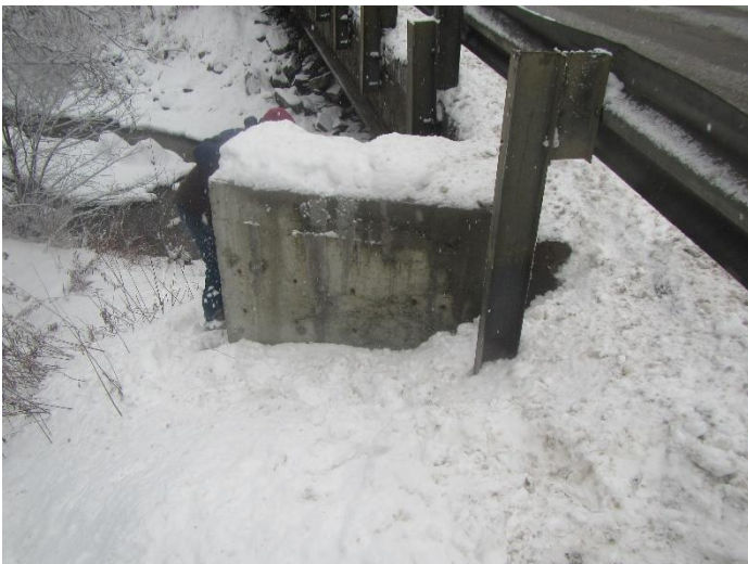
Photo 11 - Erosion behind Wingwall No. 4.
