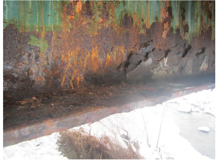
Photo 8 - Typical Girder No. 2 and 3 corrosion and section loss. Top Flange is Similar.
