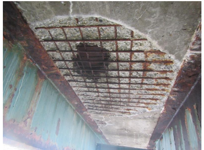
Photo 4 - Full depth hole and adjacent spalling with exposed reinforcing in deck between Girder Nos. 1 and 2, near Abutment No. 1
