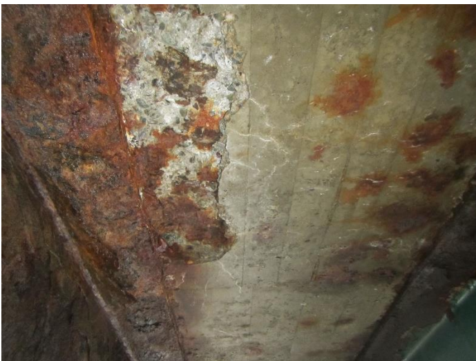
Photo 5 - Deck Underside Between Girder Nos. 2 and 3. Spalling, delaminations, and cracking with efflorescence.
