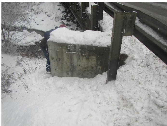
Photo 11 - Erosion behind Wingwall No. 4.
