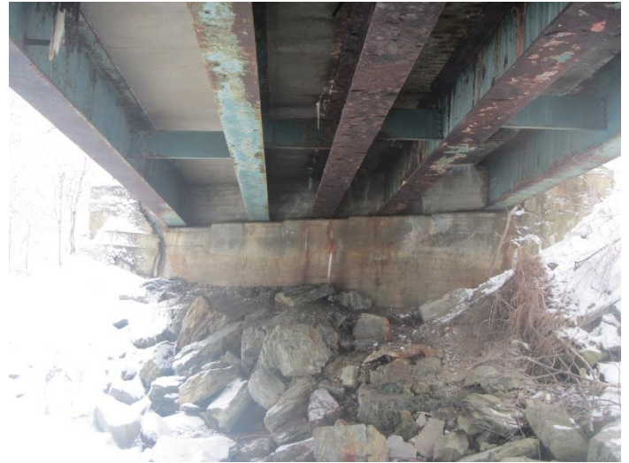
Photo 2 - Abutment No. 1 Elevation and Underside. Note the difference in deck concrete left and right of Girder No. 3
