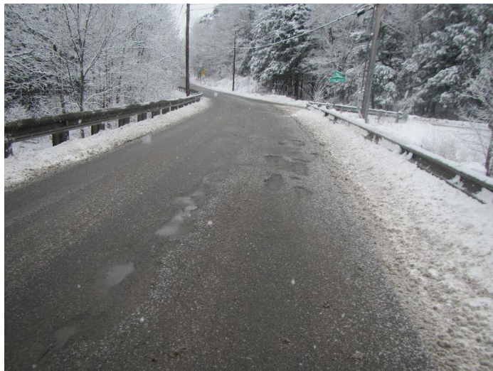
Photo 7 - Typical top of bridge, facing east. Note heavy pavement delaminations and potholes in easbound lane.
