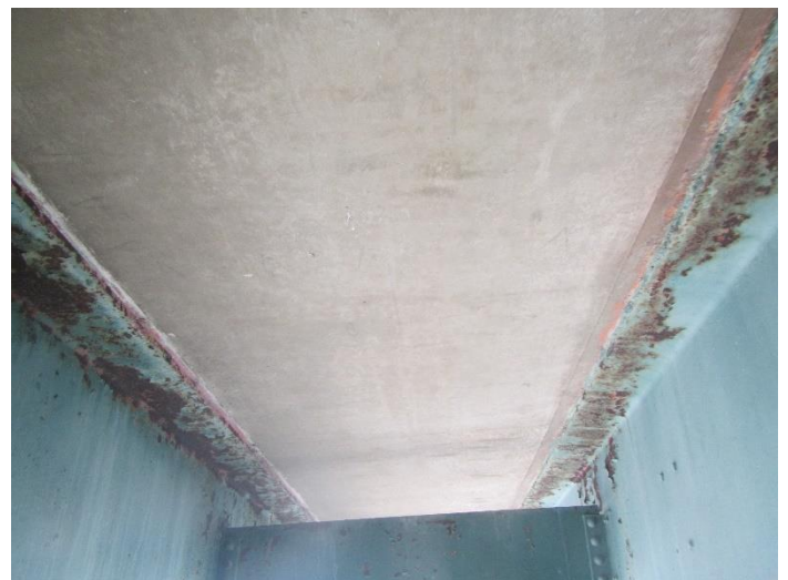
Photo 6 - Typical deck underside condition between Girder Nos. 4 and 5.
