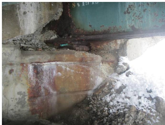
Photo 10 - Abutment No. 2 at Girder No. 5. Spalling to bridge seat and backwall, undermining the bearing.
